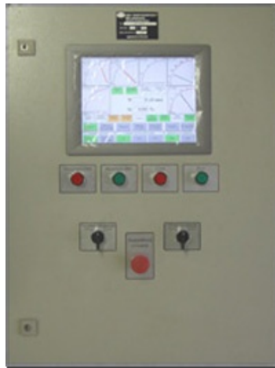
Fig. 1 SUDG-1000-6,3 control system for 8CH32/40 diesel engine (OJSC "RUMO", Nizhny Novgorod) GSD-1000-1000 generator (OJSC HC "Privod", Lysva)
